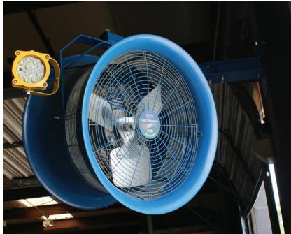
Attached to a dock fan
